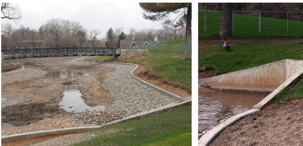
Left: Liberty Park Lake, following reconstruction of concrete wall and replacement of cobble along banks
